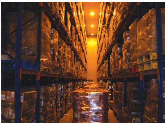
Lights - 400W HPS Illumination at floor level - 250 lux
